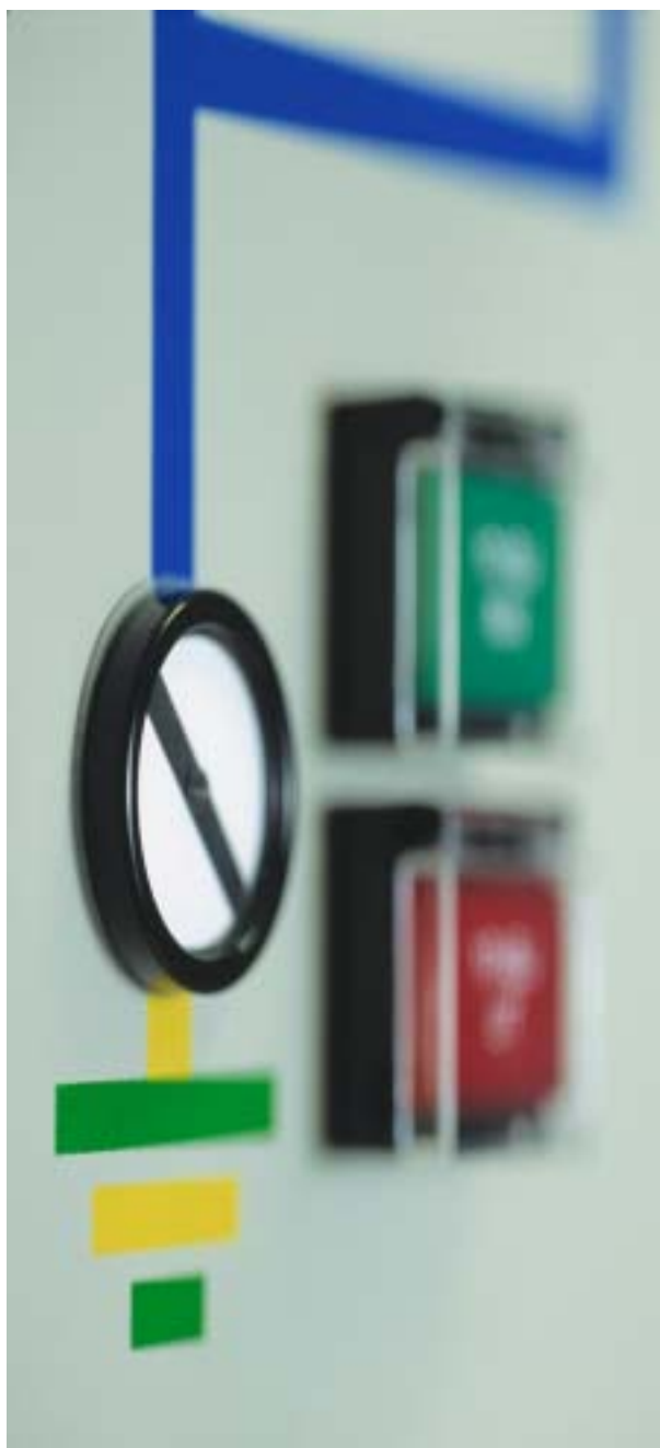
Control panel. Photo: Trond Isaksen
